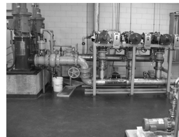
Raw Water Lift Pumps and Prefilters
