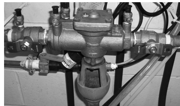
Backflow Device Used to Prevent Cross Connection Contamination.
